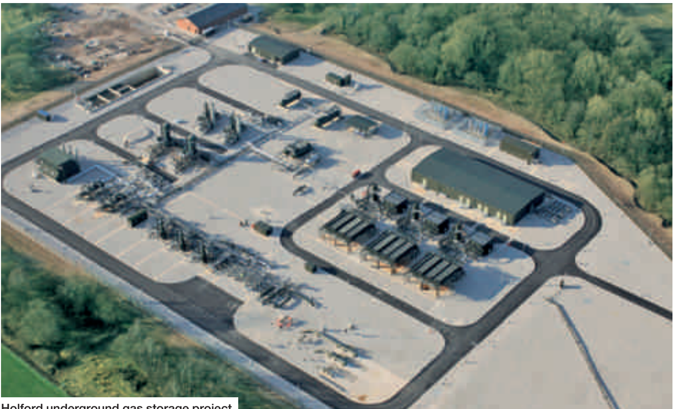
Holford underground gas storage project
